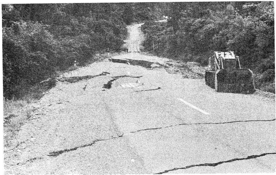
S.H.G R.M. 193.80 M . Coal Creek approaches : Road subsidence
