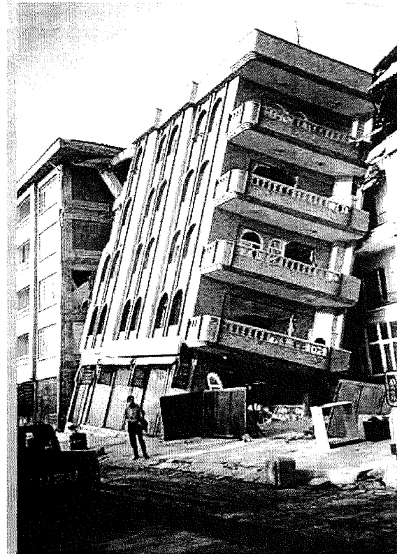
Figure 1a: Rigid body response of buildings with stiff shallow foundations to earthquake-induced liquefaction following the August 17 1999 Kocaeli earthquake in Turkey (courtesy Earthquake Engineering Field Investigation Team, UK).
